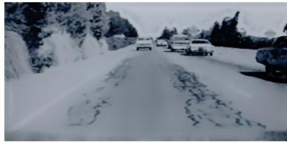
(b) Cracks in wheel tracks
