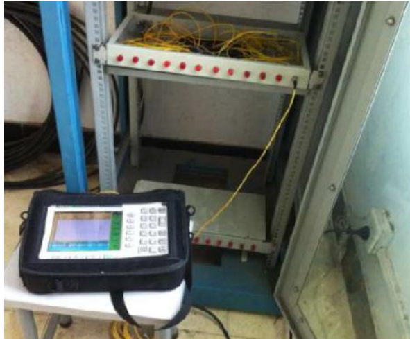
Figure 3: OTDR connected to fiber under test
