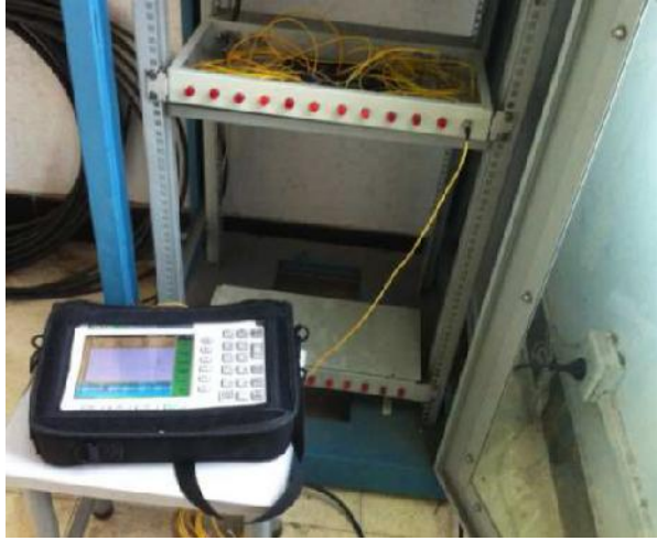
Figure 3: OTDR connected to fiber under test
