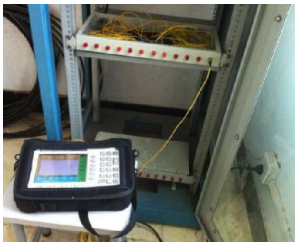
Figure 3: OTDR connected to fiber under test
