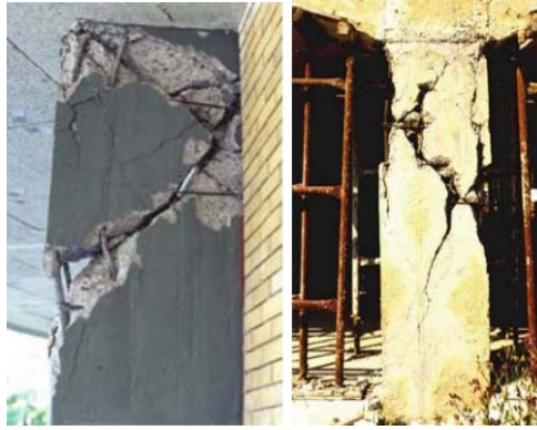
Fig. 1. Shear failures of columns [6].
