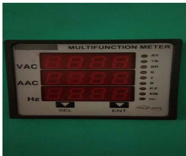
Fig. 5. Multi-function meter for ohmic heating system.
