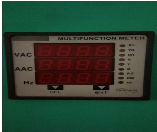
Fig. 5. Multi-function meter for ohmic heating system.
