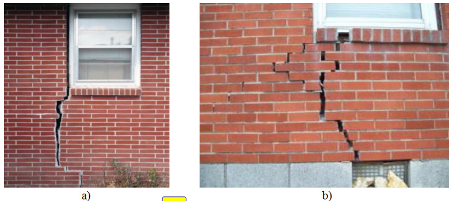
Fig.1. Building damage: produced by a) shrinkage[11], b) swelling [12].
