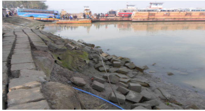
Fig.2. Photographic view showed the severe erosion prone area at Lebukhali Point of Payra River.
