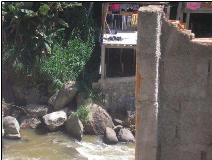
Photo 1: Irregular dwellings built along the river. Source: Authors.
