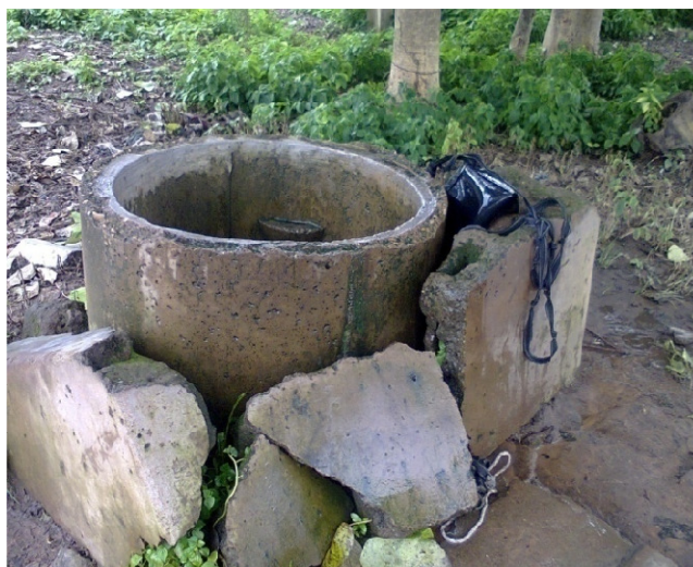
Plate 6: A Dilapidated Hand-dug well at Kueke, Surulere LGA (Source: Author's fieldwork, 2012)
